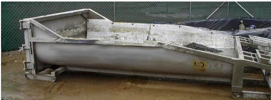
Plate 4-6 - Typical washout facility
