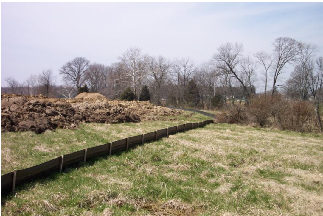
Plate 4-2 - Typical silt fence usage
